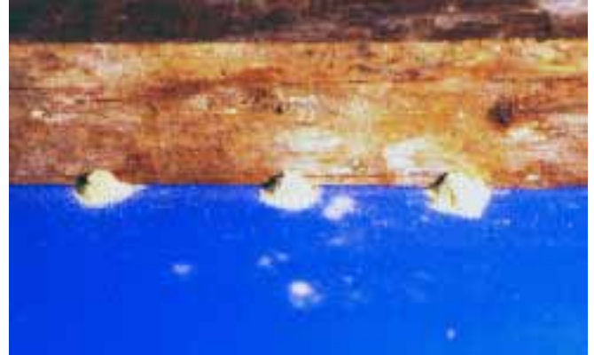
Figure 3. Larvae of powderpost beetles can reduce susceptible timber to a fine flour-like powder.
